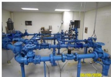
Existing Process Piping
