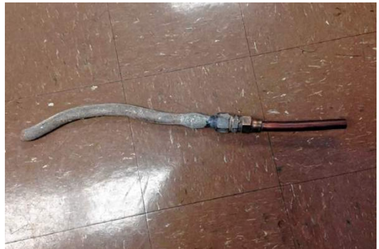
Lead Pipe Example
