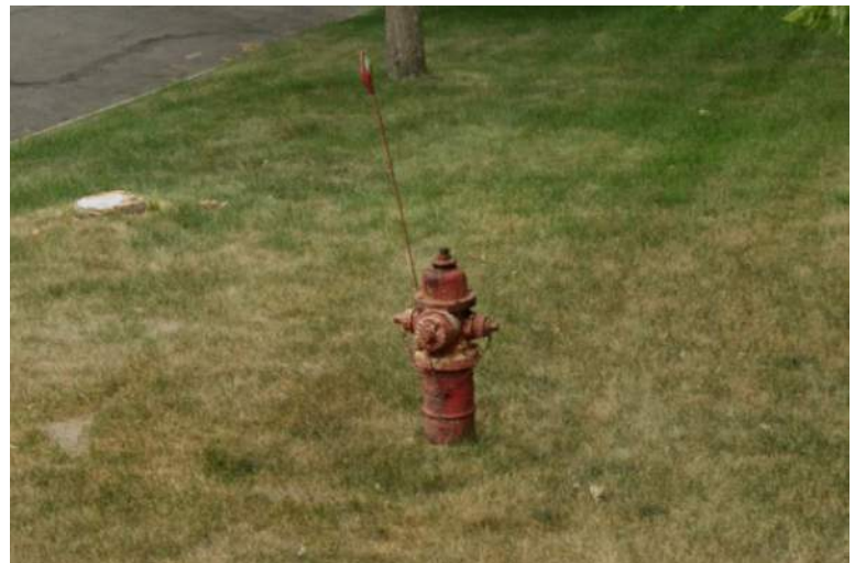
Existing Fire Hydrant
