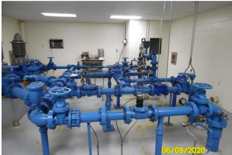
Existing Process Piping
