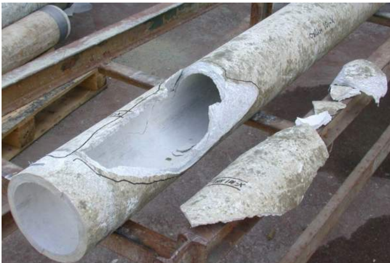
Example ACP Pipe Failure
