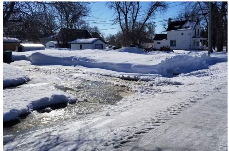
4th Ave south of Linden Street - Drainage Issue
