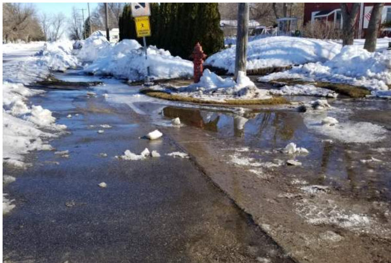
Spruce Street and 5th Ave - Drainage Issue
